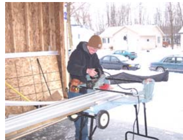
Austin Nelson cuts soffit to finish the eaves on the trades house.
